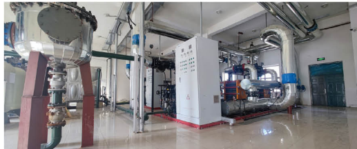
Integrated Intelligent Heating System
