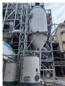
Completion Effect of Evaporator and Supporting Water Tank
